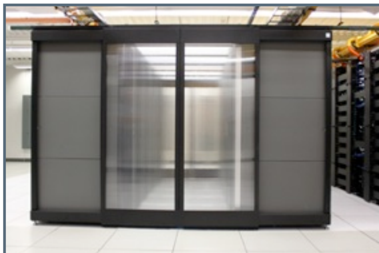
Cold Aisle Containment
